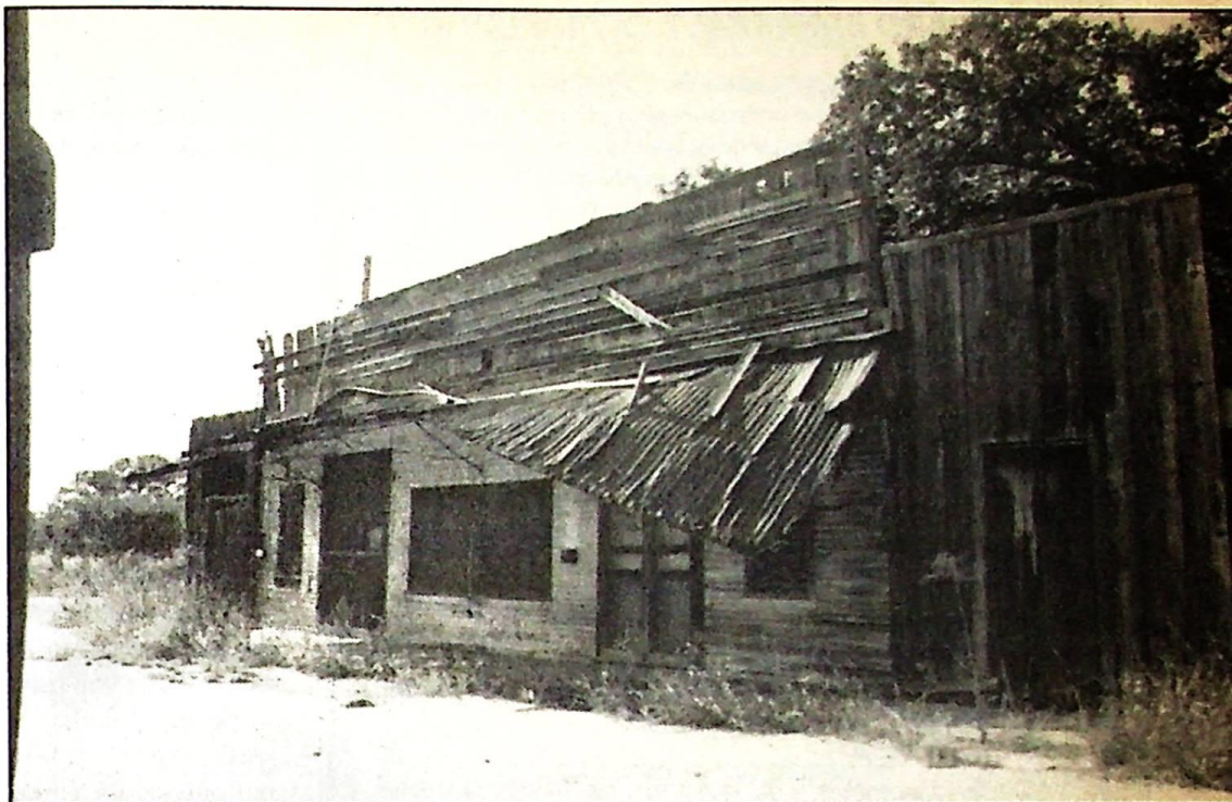
ABOVE: TODAY ONLY A STORE AND POST OFFICE REMAIN OF WHAT WAS ONCE A LITTLE VILLAGE WITH TWO CHURCHES, BLACKSMITH SHOP, DRUGSTORE, BARBER SHOP AND TWO STORES. ONE OF MY FAVORITE DILAPIDATED BUILDINGS STILL STANDS HERE. APART FROM THAT THERE ARE A FEW RESIDENCES AND NOTHING ELSE. OPPOSITE: ONE OF SEVERAL ABANDONED GAS PUMPS IN FREDONIA.
